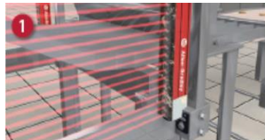
1. Light curtain has buildup of dirt reducing sensing field.
